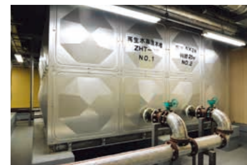
貯水槽 Water tank
